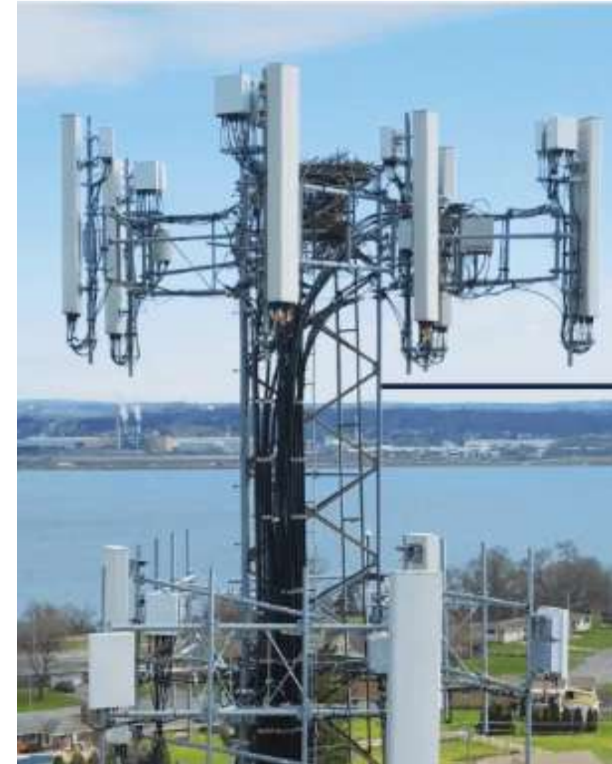
Example of Communications Tower with Multiple Radomes
